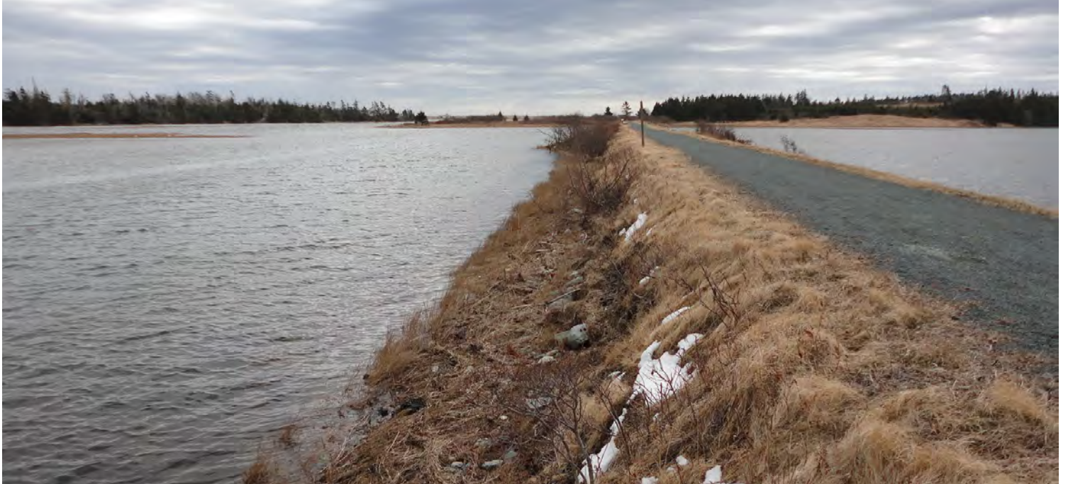
Ongoing erosion with the majority of embankments slopes < 1:1, with isolated areas where the trail width was compromised – May 2012
