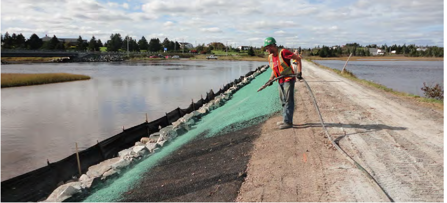
Common material placed to restore 2:1 embankment slope; installed TRM (Enkamat 7020); and ongoing application of hydraulic mulch – October 2012
