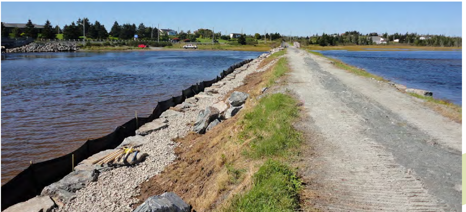
Silt control fence installed; armour rock placed along the restored toe of slope; 25 mm clear stone placed between the armour rock and the existing toe of slope – September 2012
